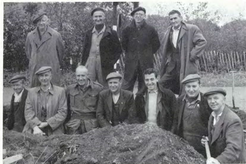
The rain which was falling when this picture was taken was not enough to damp the spirits of this group from Wrexham and Legacy Mains staff who were busy taking electricity to a new housing area at Marford. They are, left to right (back row): Messrs. J. D. Roberts (Labourer), F. Bolton (Chargehand), H. E. Smith and T. Price (Labourers). Front row: Messrs. O. Bennet, R. B. Bellis, N. Hatton, J. L. Griffiths, R. C. Harrington, C. Griffiths, and J. Masterton (Labourers).
